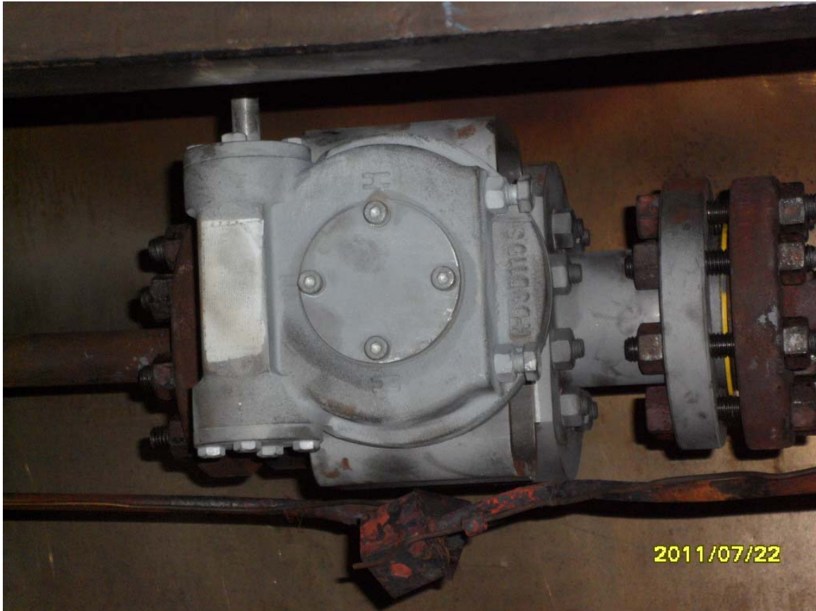
Valve Prior to Test
