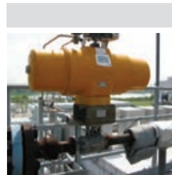
This ValvTechnologies' valve is installed in a cogeneration facility on the Gulf Coast. The application pictured is a vent valve located in the reheater section of the HRSG.
