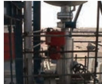
Pictured above: This Electronic Relief Valve (ERV) was installed to provide protection to the safety relief valves, which if operated could cost the plant thousands of dollars in replacement.
