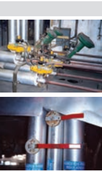
Pictured above: The function of the boiler drain and vent valves is to drain the boiler for maintenance outages. The valves are always closed when the boiler is in operation and must remain absolutely leak free while the plant is online – to ensure plant efficiency.
