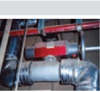
Pictured right and above are boiler feed pump recirculation valves. These ValvTechnologies XACTROL models have been in successful operation for over eight years without requiring trim or packing replacement.
