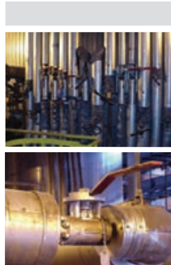
Pictured above: Main steam hot and cold reheat drain and vent valves. Steam is returned to the turbine in the hot reheat line at 1000°F (538°C), 600 psi (41 bar). The drain valves are used to heat the steam lines during start-up and discharge into condenser.
