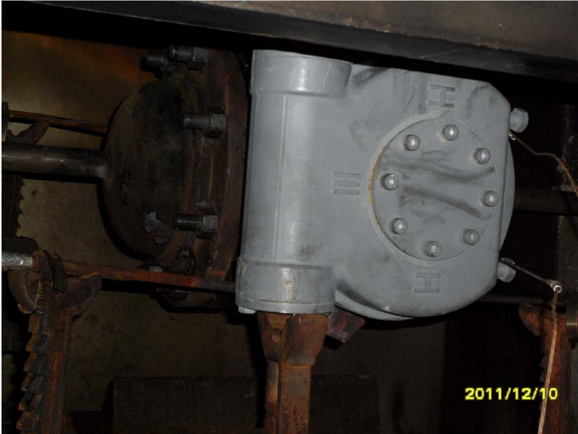
Test Valve Prior to Burn
